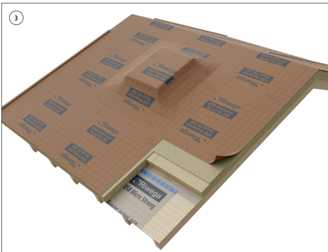
After securing the counter-batten on the edge, unfold the membrane by proceeding horizontally
