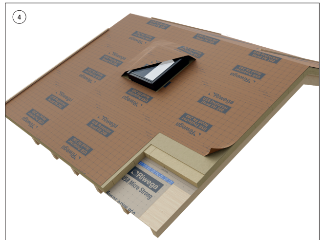
Cut the membrane and seal it around the parts emerging from the roof pitch using the appropriate accessories
